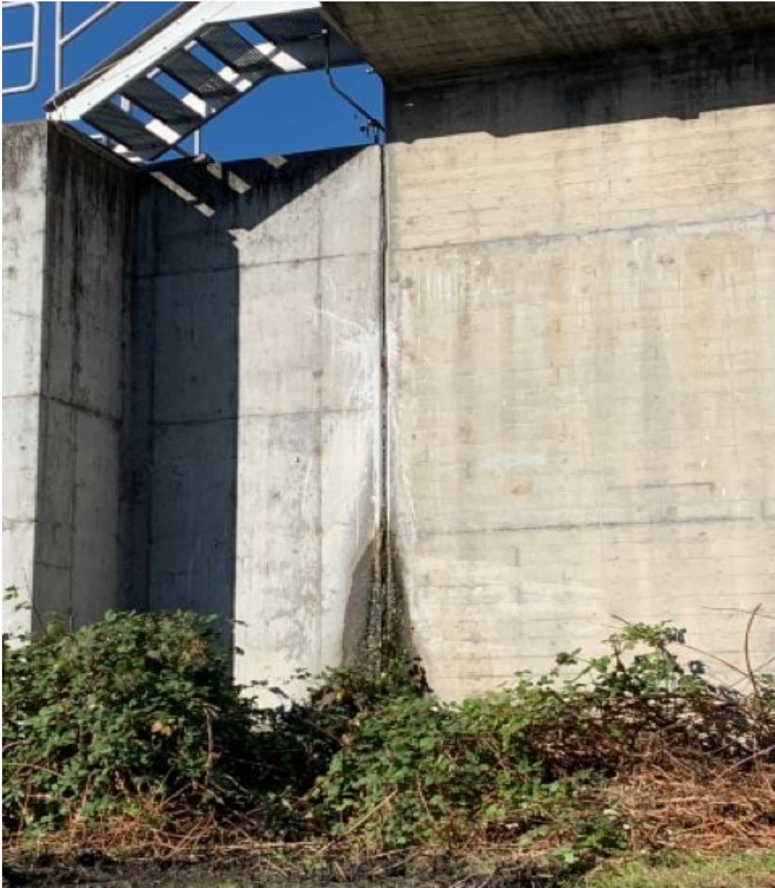
North ladder expansion joint leak. Repair this winter.
